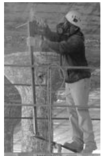
The McGovern lever in use by Paul Zangla of Laborers Local 151 Photo: Derek Lines, John Moriarty Associates
