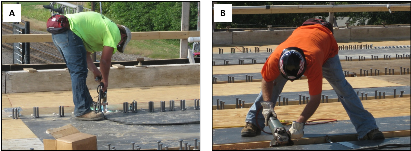
Figure 2: A – stud welding using traditional equipment; B – preparing weld locations with an angle grinder.
