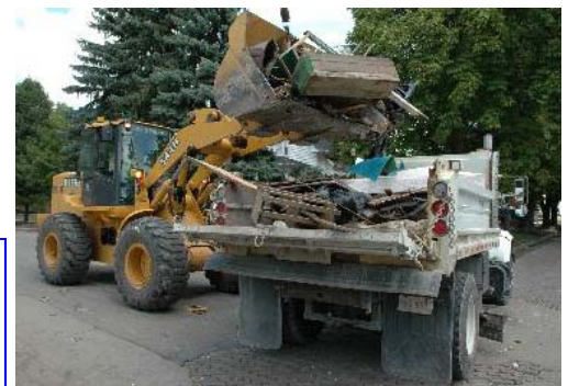
Keeping back from operations is key. Photo courtesy of FEMA
