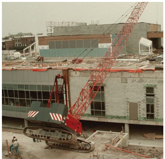
Crane tip-over at library expansion project. (Photo courtesy of The Blade/Toledo Ohio)
