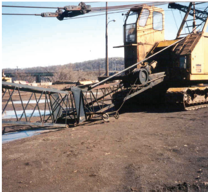
Boom collapse during crane disassembly.
