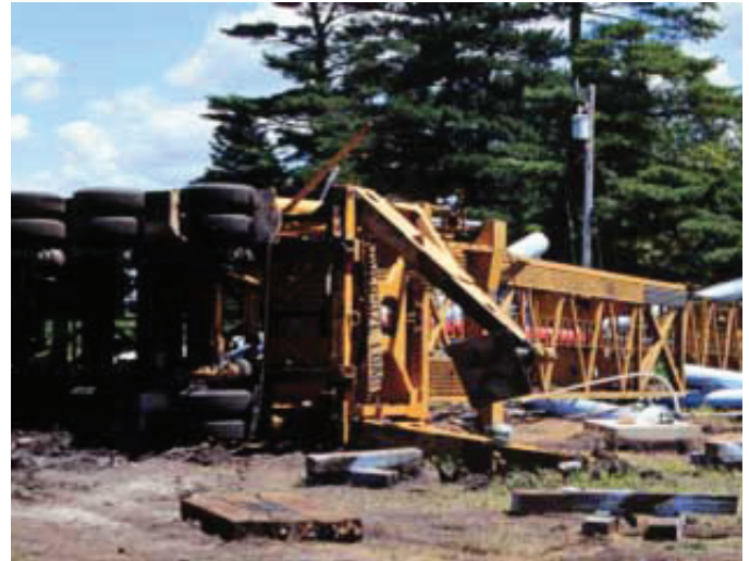
Mobile tower crane tip-over attempting to hoist water tank. (Photo courtesy of Iowa FACE Program)
